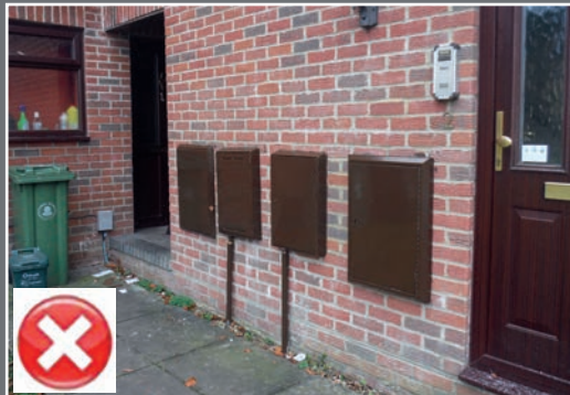
Visually dominant meter cabinets that are unattractive features on the building and in the street scene
