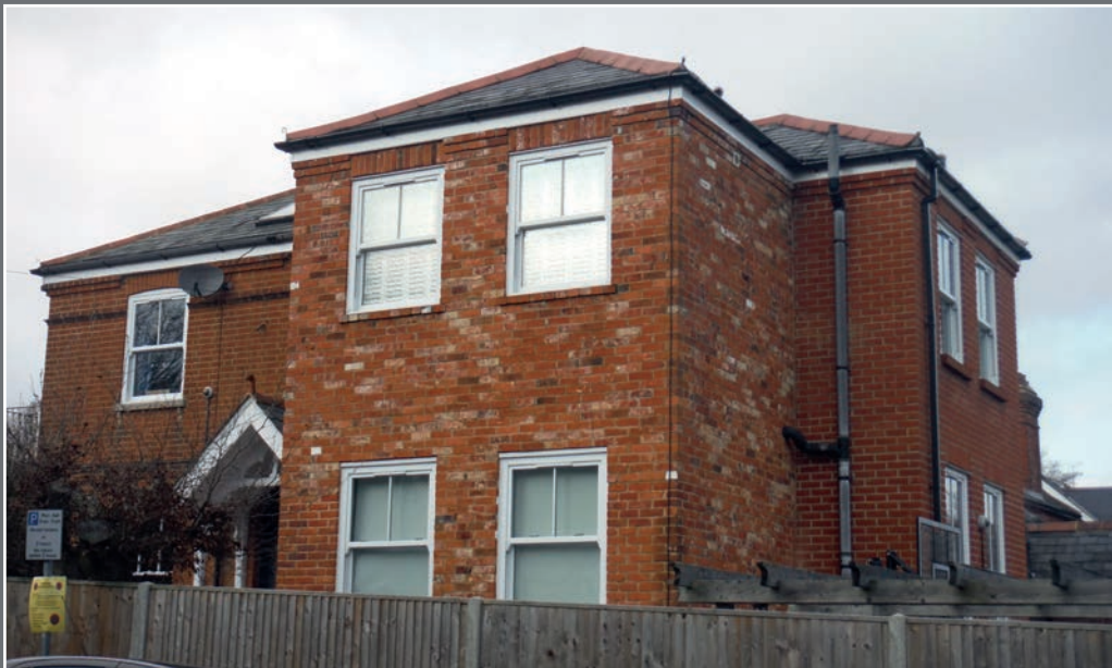
A building with two extensions that do not follow the design of the main dwelling in terms of window style, string course and brick colouring
