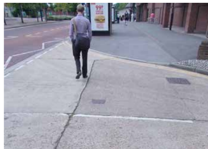
Poor quality surface materials
