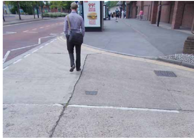
Poor quality surface materials
