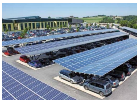
Figure 5.16: An example of a solar carport 187
